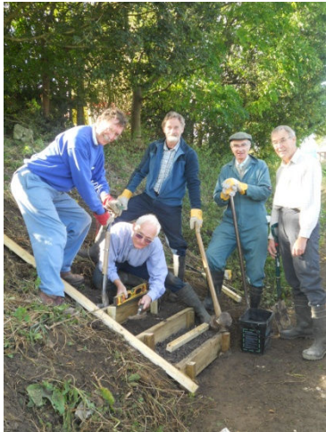
Volunteers from the local Ramblers group helped build steps from the White Horse viewing area
